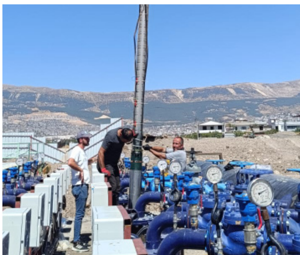
The water is distributed through a 12 km long pipeline.
