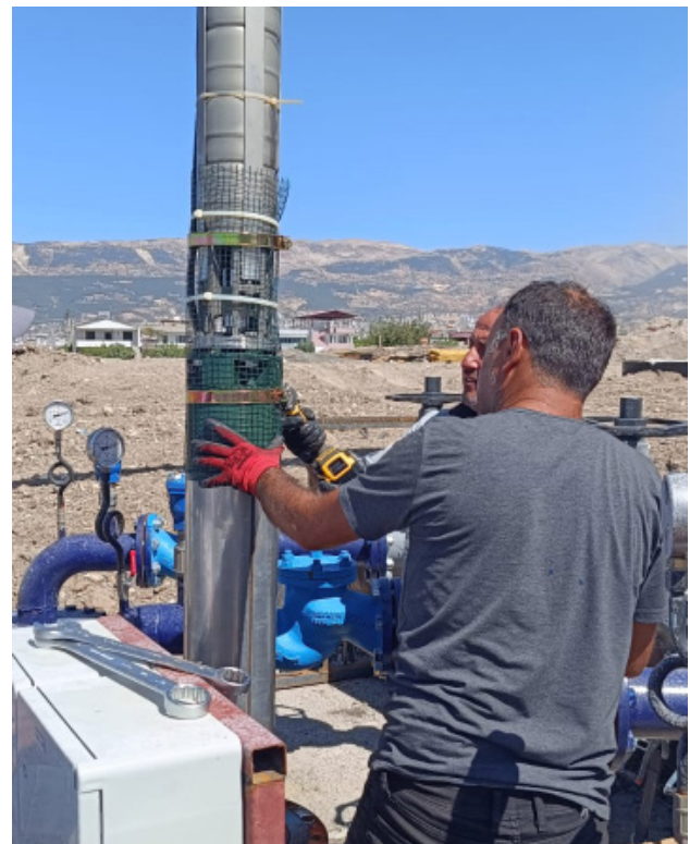
22 stainless steel submersible pumps and motors from İmpo pump the water.
