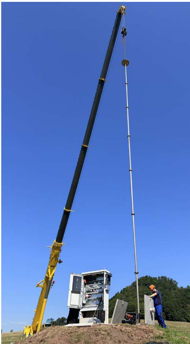
The pump system is located at a depth of 25 metres.
